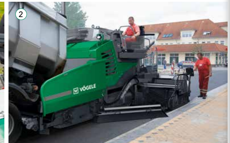
2 A very low spray pressure of no more than 3 bar allows absolutely uniform spreading of bitumen emulsion and a clean result when spraying along kerbs.
